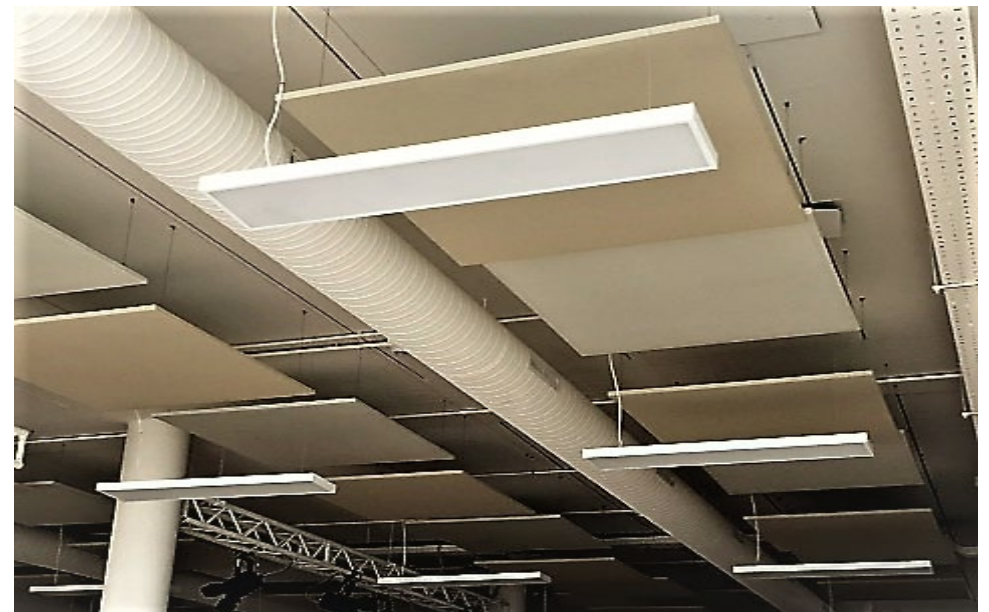
Gadames 57 – specific sound-absorbing panels
